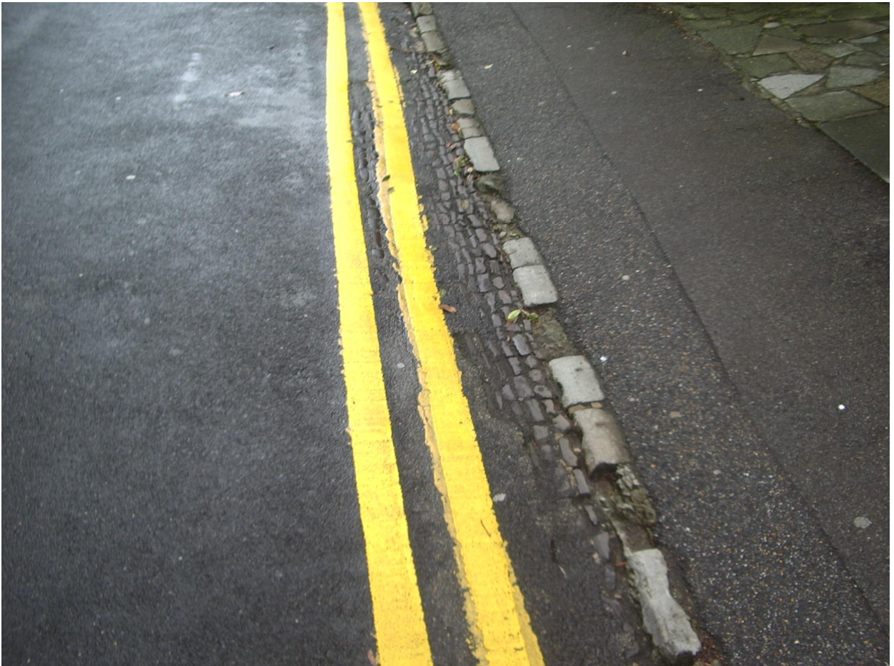
Attractive ironstone setts and stone kerbs in Hollybush Lane over painted with harsh and thick double yellow lines
