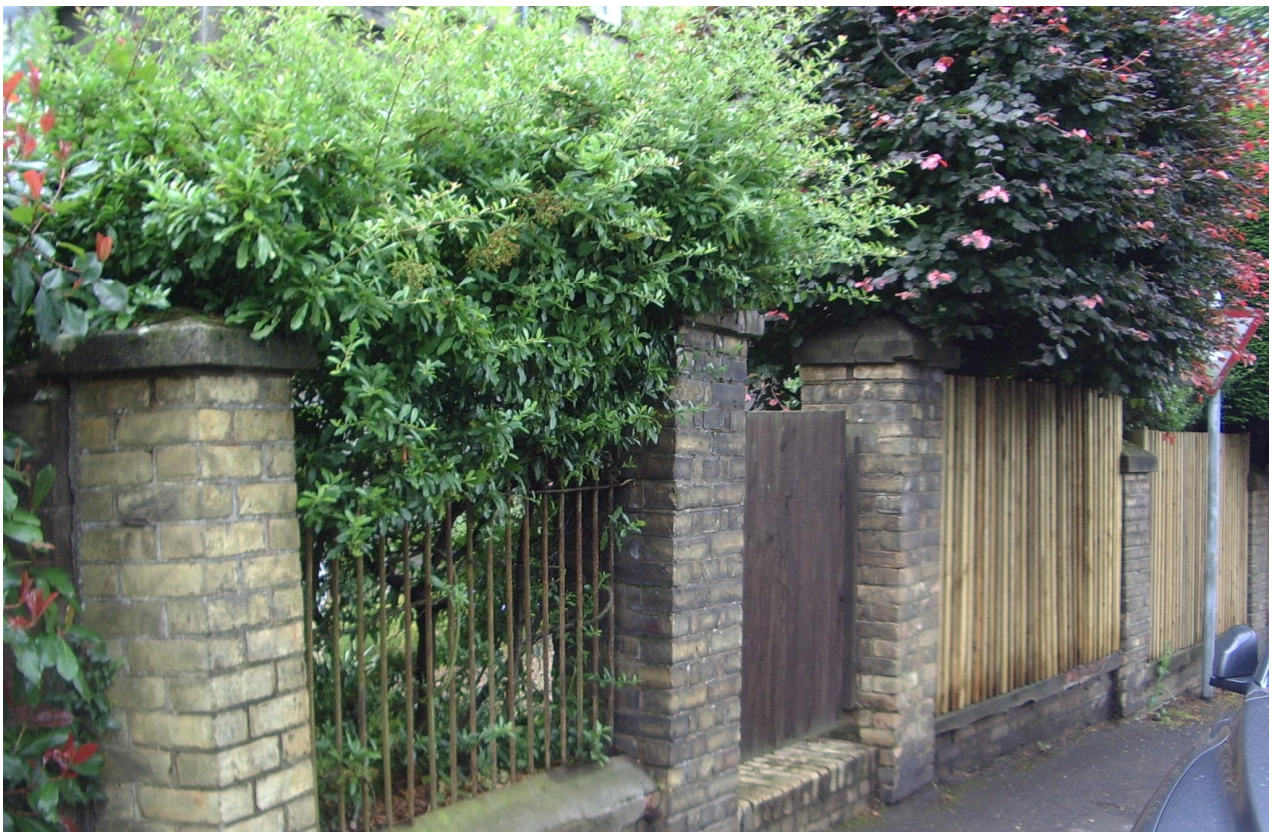
Wall in Bayham Road – note loss of historic railings
