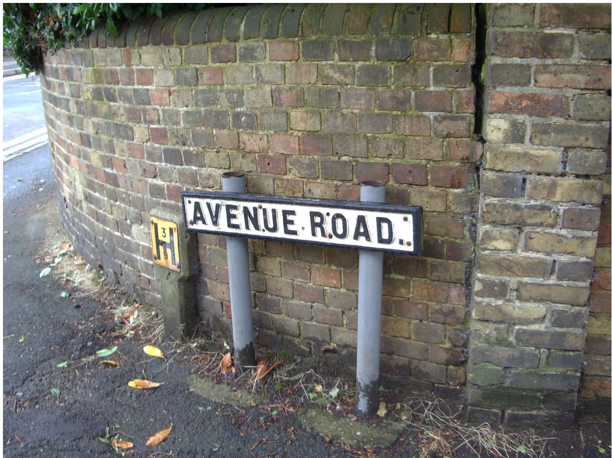
Attractive old road sign compromised by modern, standard and inappropriate posts. Also note poor quality highway maintenance.
