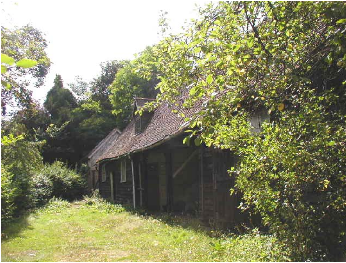
34. Fine eighteenth century barns remain mainly low-key and rural in appearance. These buildings are quite delicate and have already suffered some collapse.
