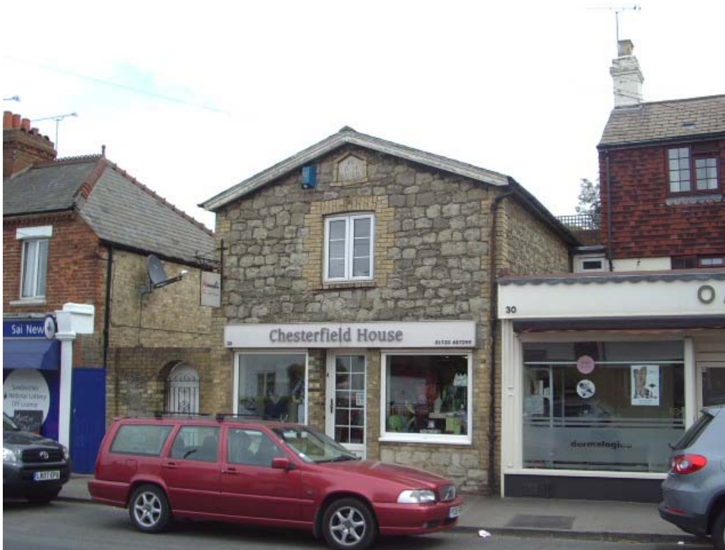
56. UPVC windows are poor quality and do nothing to highlight the unique quality of the Conservation Area
