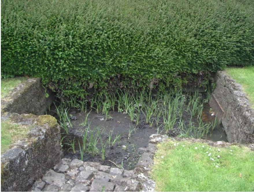
17. Evidence of series of linked ponds – this is crucial to the history of the Conservation Area
