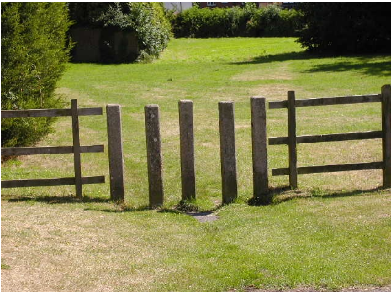
13. Weathered concrete bollards – a timber wheelchair and pushchair friendly gate might be more appropriate as these bollards block the footpath for these users. Any replacement should be agreed with Conservation.
