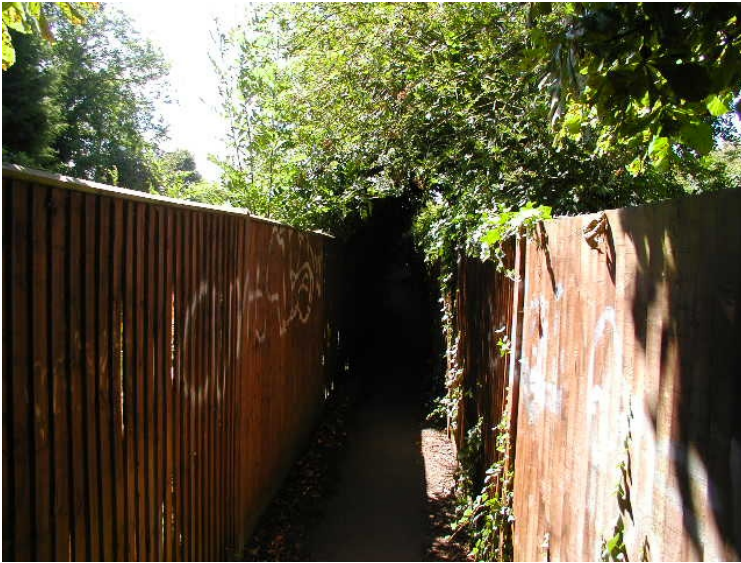
57. Note inappropriate close boarded fence and graffiti. A footpath such as the one above should not have close boarded fencing as this does attract graffiti. Prickly bushes or shrubs and trees would be a preferable option.
