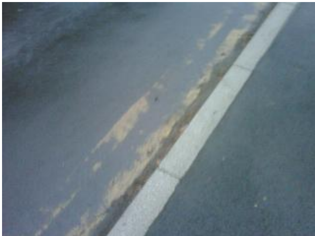
Unnecessary thick yellow lines in Oakhill Road. will be repainted as budgets allow.
