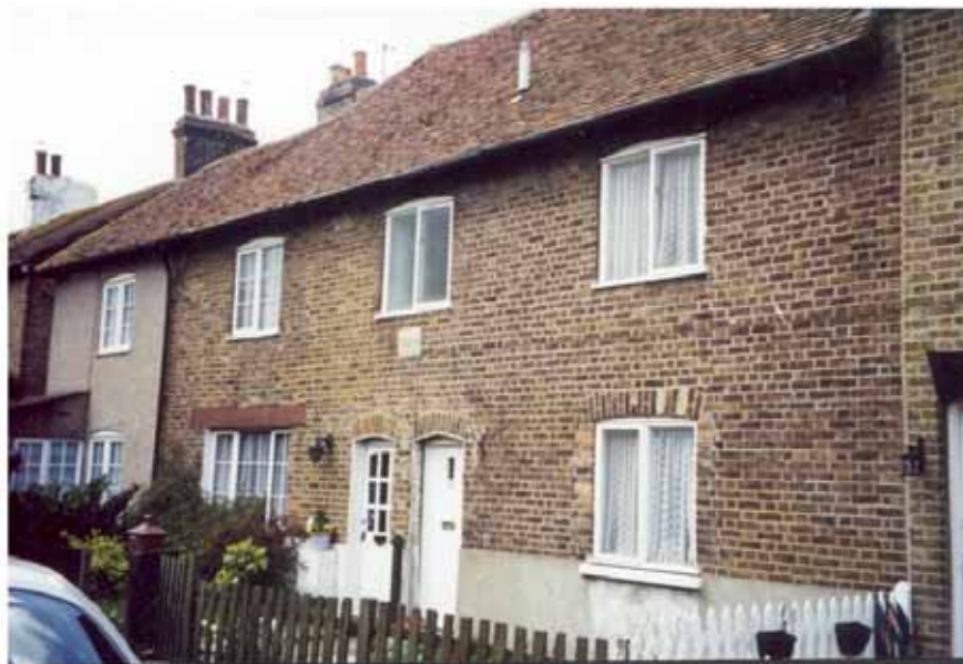
Fig 66: Unsympathetic alteration of window opening
