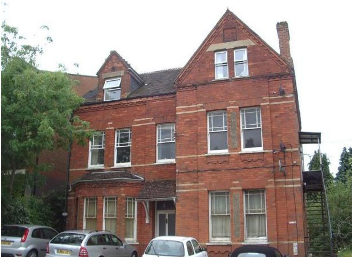
Lack of maintenance and UPVC windows in Granville Road house
