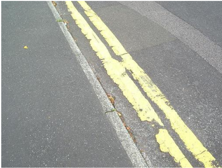
Unnecessary badly painted thick yellow lines in Granville Road.
