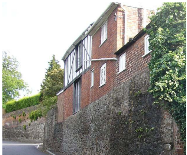
Soil pipe on Bank House
