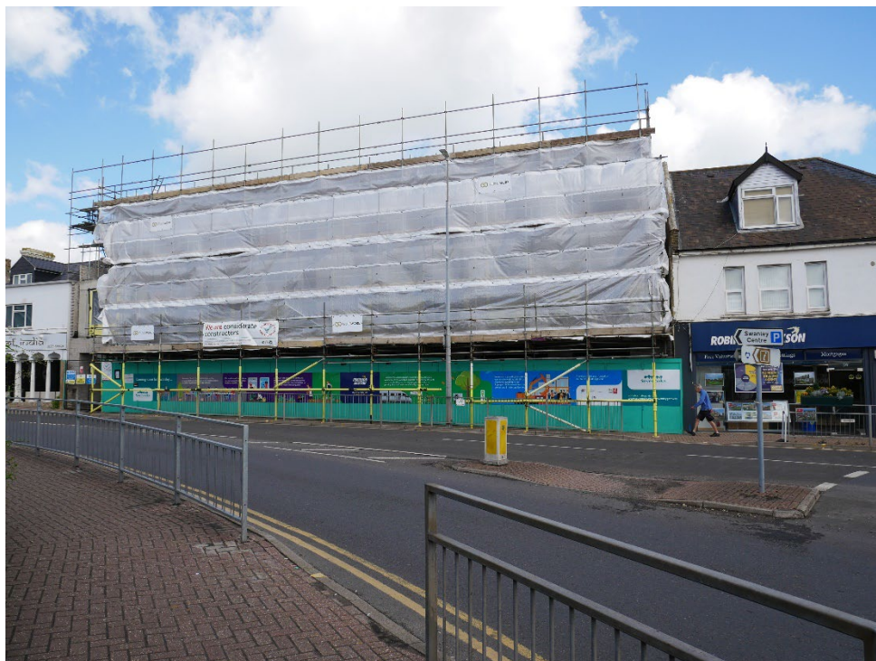
The High Street Looking from the lower roundabout showing the new three storey mixed use development under construction.
