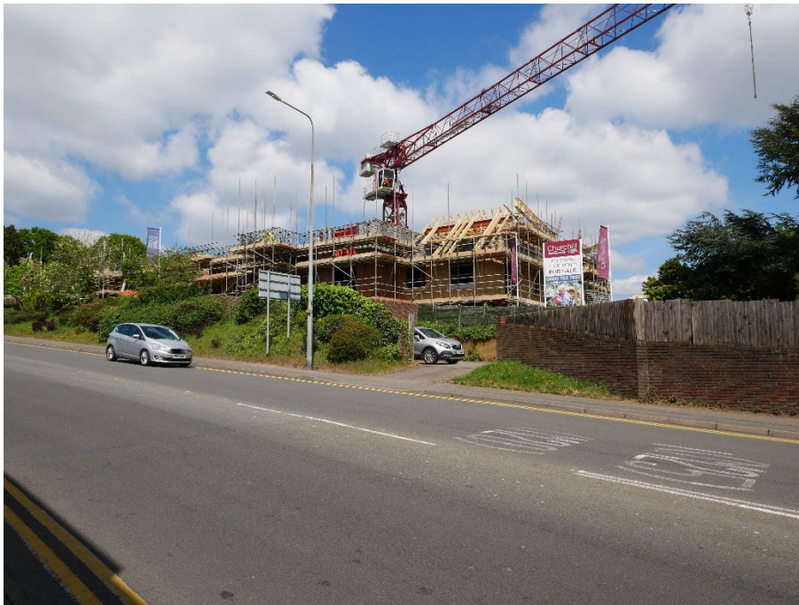
A view of the three-storey private retirement development under construction in Bartholomew Way.
