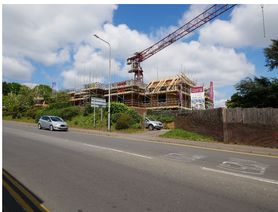
A view of the three-storey private retirement development under construction in Bartholomew Way.
