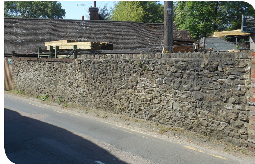
Inappropriate pointing to some ragstone walls
